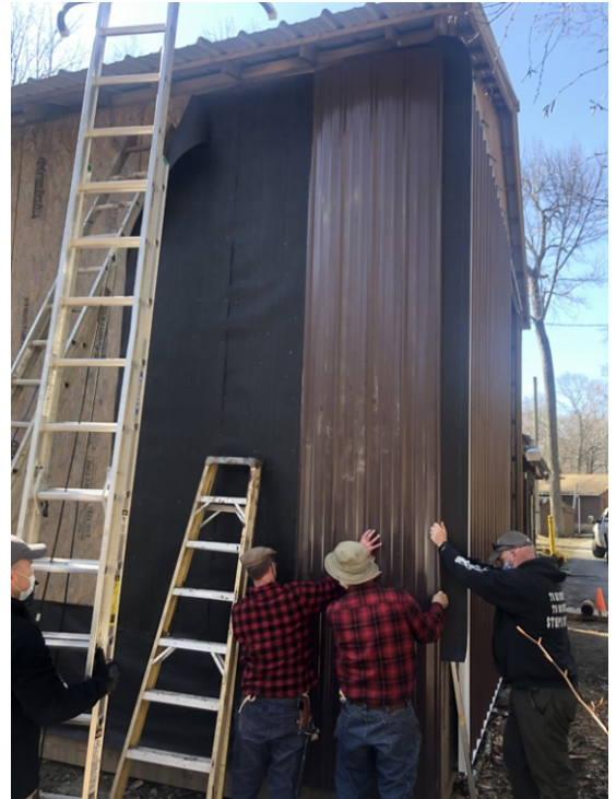
At last! Siding going up on the Pole Barn Chris Johnson, Mark O'Connor, Brian Goodrich and Ranger Frank
